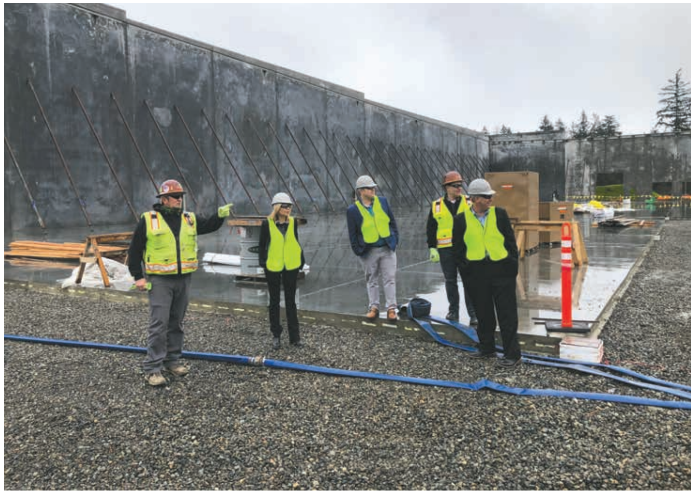
Clayco Project Superintendent David Cordray, left, in charge of the construction of the Lowe's Home Improvement regional distribution center just off Interstate 5 near Winlock, points out details of the 1.2 million square foot project during a tour earlier this year. Next to him is Lisa Goodman, The Benaroya Company marketing director, Lewis Economic Development Council External Relations Eric Sonnenberg, a Clayco project manager, and LEDC Executive Director Richard DeBolt.
